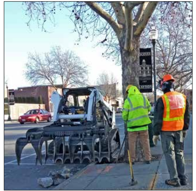
Main Street trees and roots inspected
